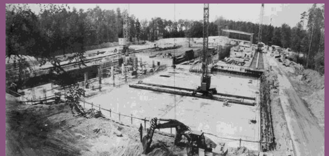
Construction works of GSI buildings at the beginning of the 1970s: In the foreground the experimental halls are being built, in the background facilities for the UNILAC accelerator (Photo: A. Zschau, GSI)
